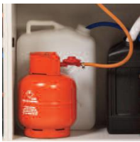
Water management system and gas bottle storage
